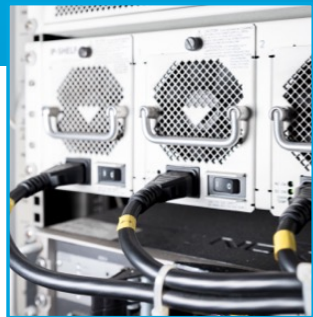
Power Supplies | UPS
